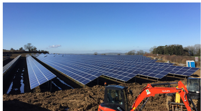
A 2.34MW solar array at Wilmington Farm, installed by Bath and West Community Energy. Photo: Bath and West Community Energy. http://www.bwce.coop/projects/wilmington-farm/
